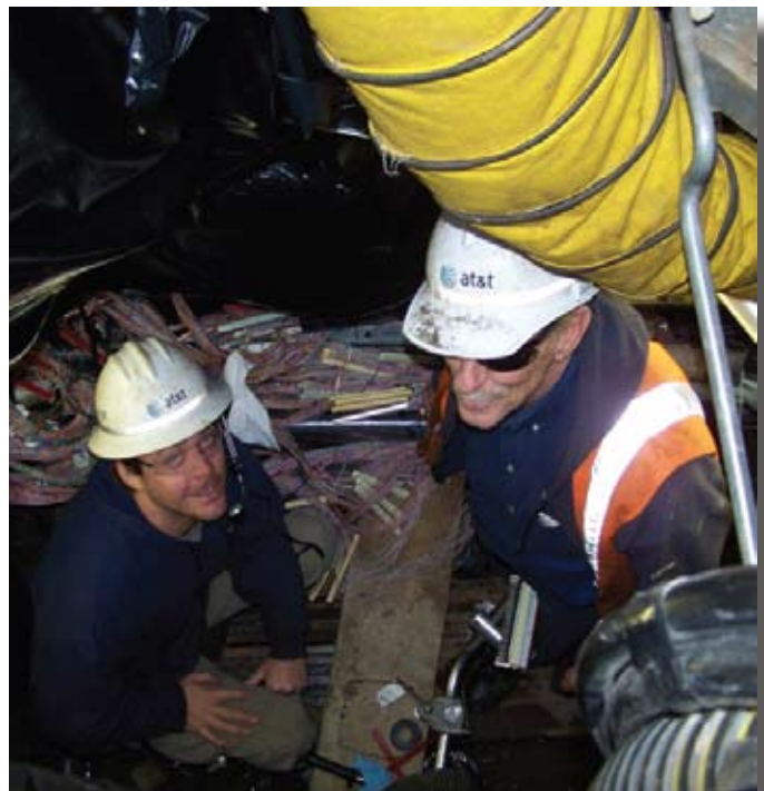
Tim Stacy and Terry Saunders are hard at work in a manhole splicing a cable on Route 30 in Frankfort.
